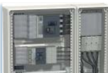
630A and 250A supply modules upstream and downstream from the busbar
