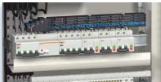
Supply of switchgear before distribution by Multiclip 80A.
